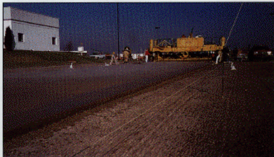
Figure 3. Before placing the overlay, the contractor rotomilled and air blasted the asphalt surface to improve bond with the concrete overlay.
