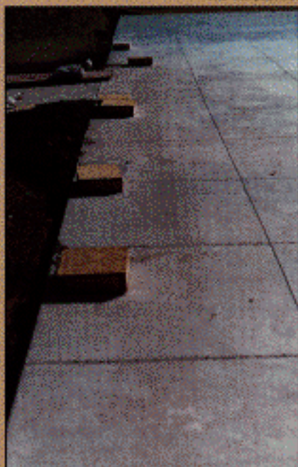
Researchers placed strain gauges to measure stresses in the concrete in the ultra-thin sections of the Spirit of St. Louis apron. Note the short joint spacing used in the ultra-thin design.
