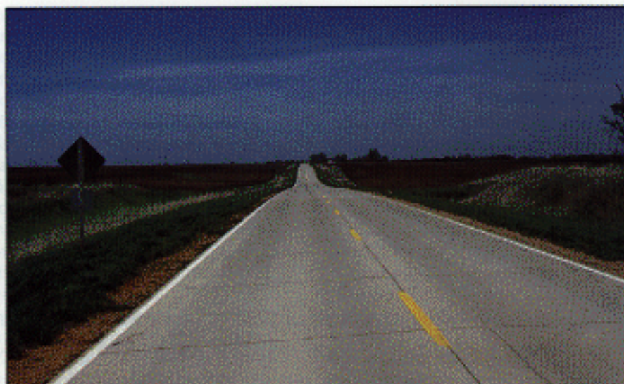
Most whitetopped pavements in Iowa have performed well. This 1990 photo shows a whitetopping completed in Boone county in 1981. After nine years, the pavement shows no deterioration.
