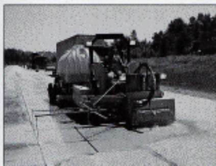
Figure 1. The machine above saws the edges of all six dowel slots at one time. The machine below saws three slots at a time. After sawing, traffic can be returned to the pavement until the fins between the sawcuts are removed.
