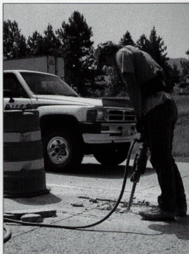
Figure 4. One technique to remove the fins is to place the jackhammer at the end of the fin and jackhammer down and along the bottom of the sawcuts. With some practice, most workers can remove a fin in two or three large pieces.
